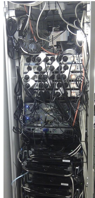
Figure 4. Smart Plugs attached to the Data Center
